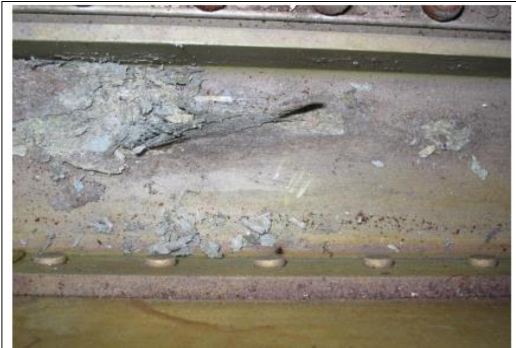
Figure 3-7: Exfoliation corrosion (Civil Aviation Authority, 2017)
