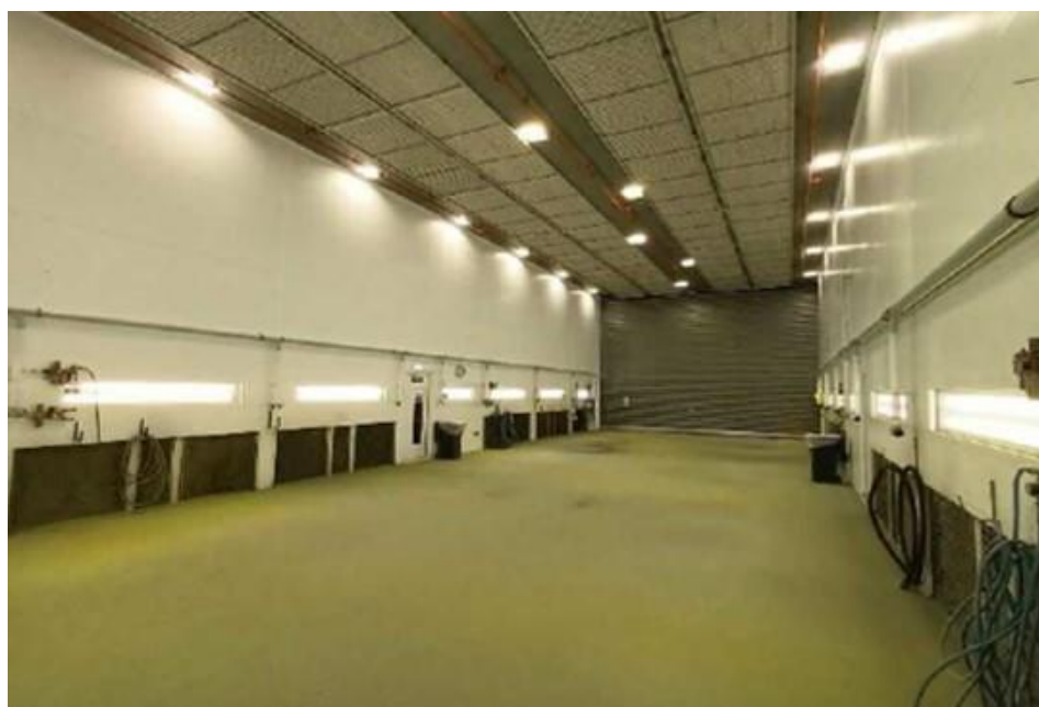
Figure VIII-4: Small spray hangar with installed side wall extraction (laminar cross flow)
