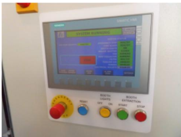
Figure 9-10: Booth extraction control panel
