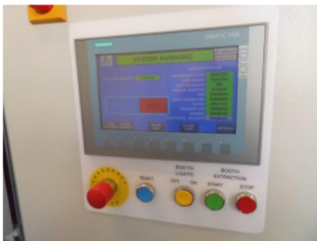
Figure 9-10: Booth extraction control panel
