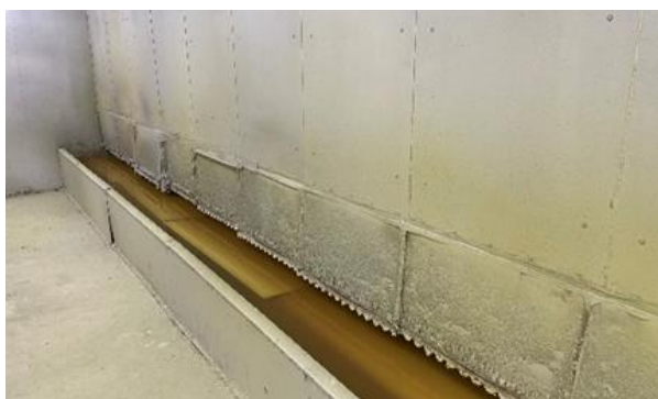
Figure VIII-2: Spray room with an installed water curtain as air abatement
