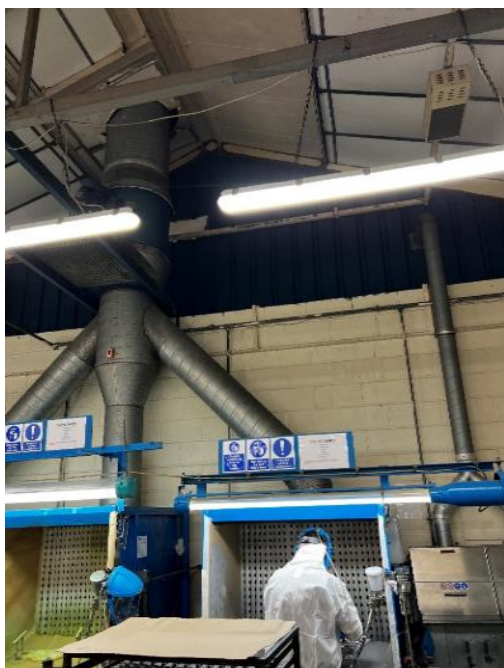
Figure VIII-1: Open spray booth where exhaust air from three booths is emitted via one stack
