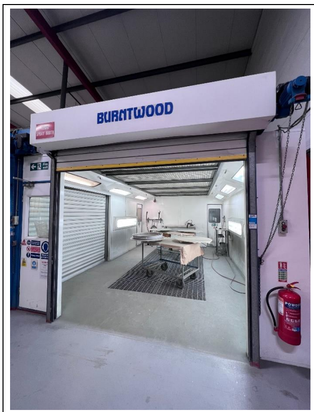
Figure 9-1: Closed spray booth
