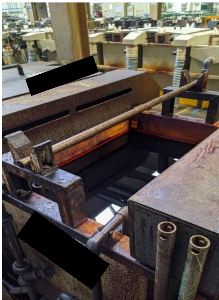
Figure 9-3: Tank equipped with air exhaust system
