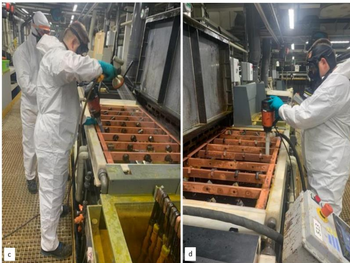
Figure 9-12: Bath emptying by transfer of old bath solution into an IBC (a) and bath cleaning with a hose and wet and dry vacuum cleaner (b, c, d)
