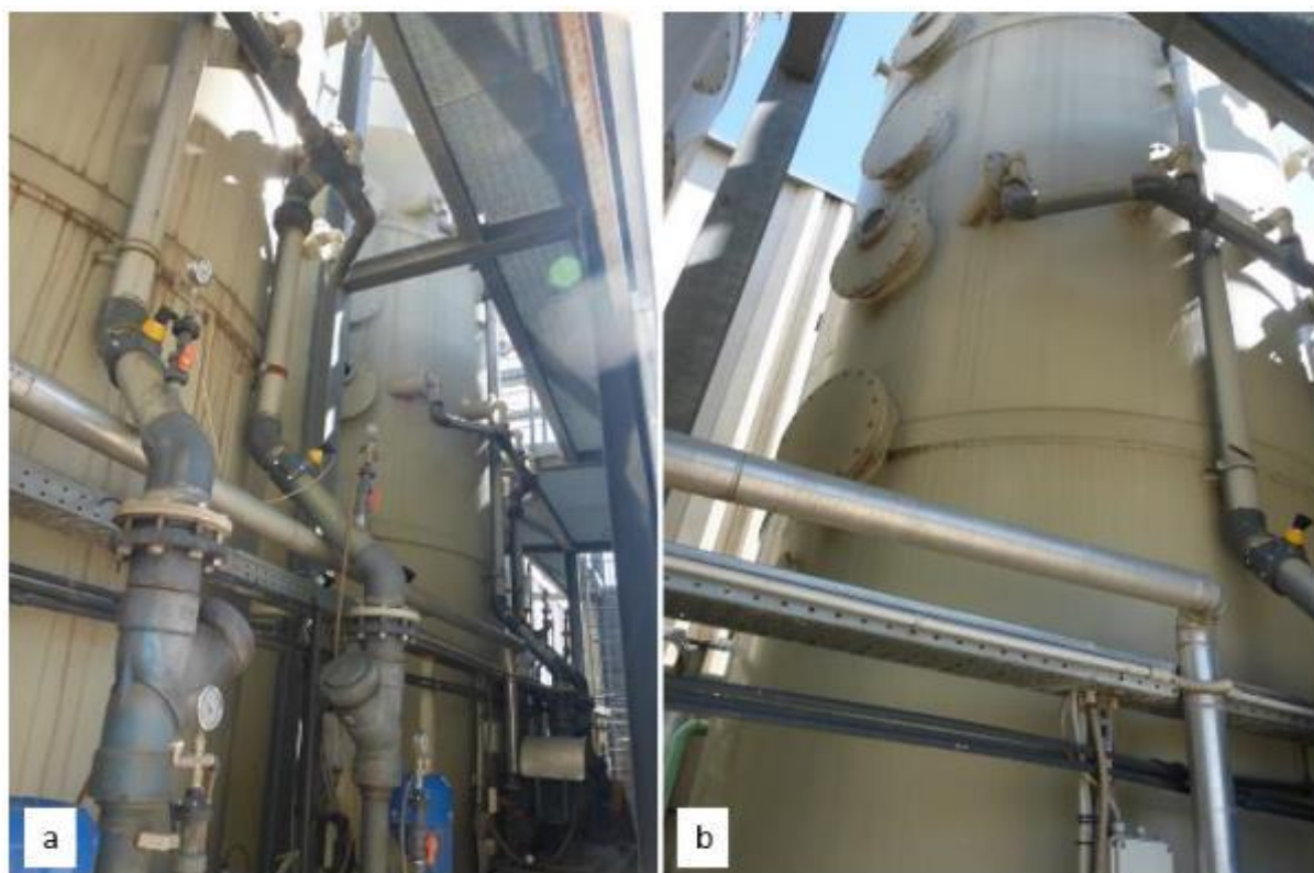
Figure 9-4: Wet scrubber (a + b)
