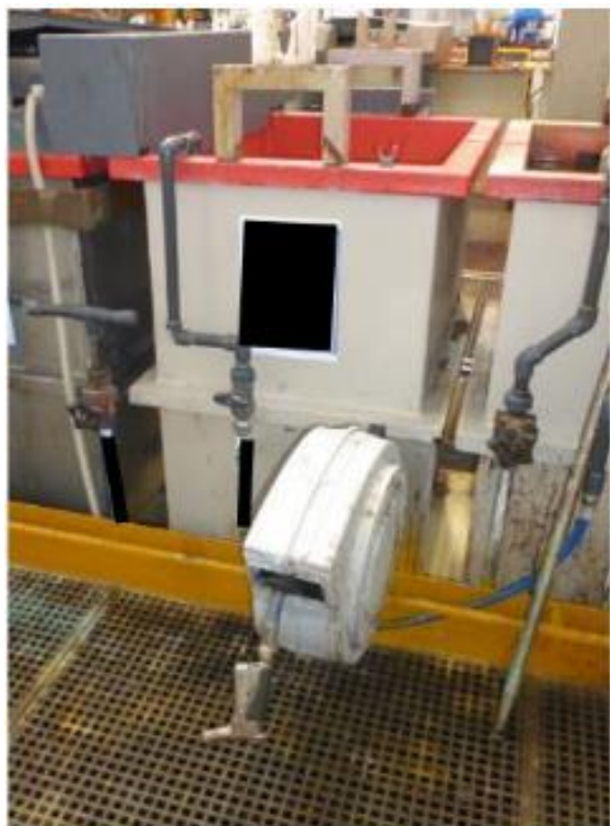
Figure 9-8: Hose for cleaning the edges of the tanks and the walkways surrounding the baths
