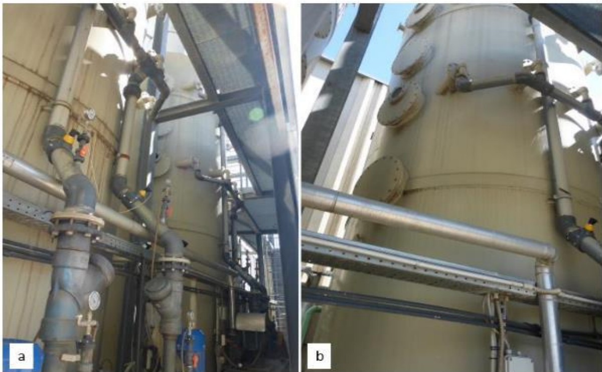
Figure 9-4: Wet scrubber (a + b)
