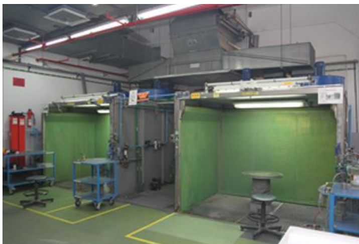
Figure 9-3: Spray booth closed at three sides and open in the front with a running water curtain on the three walls and LEV
