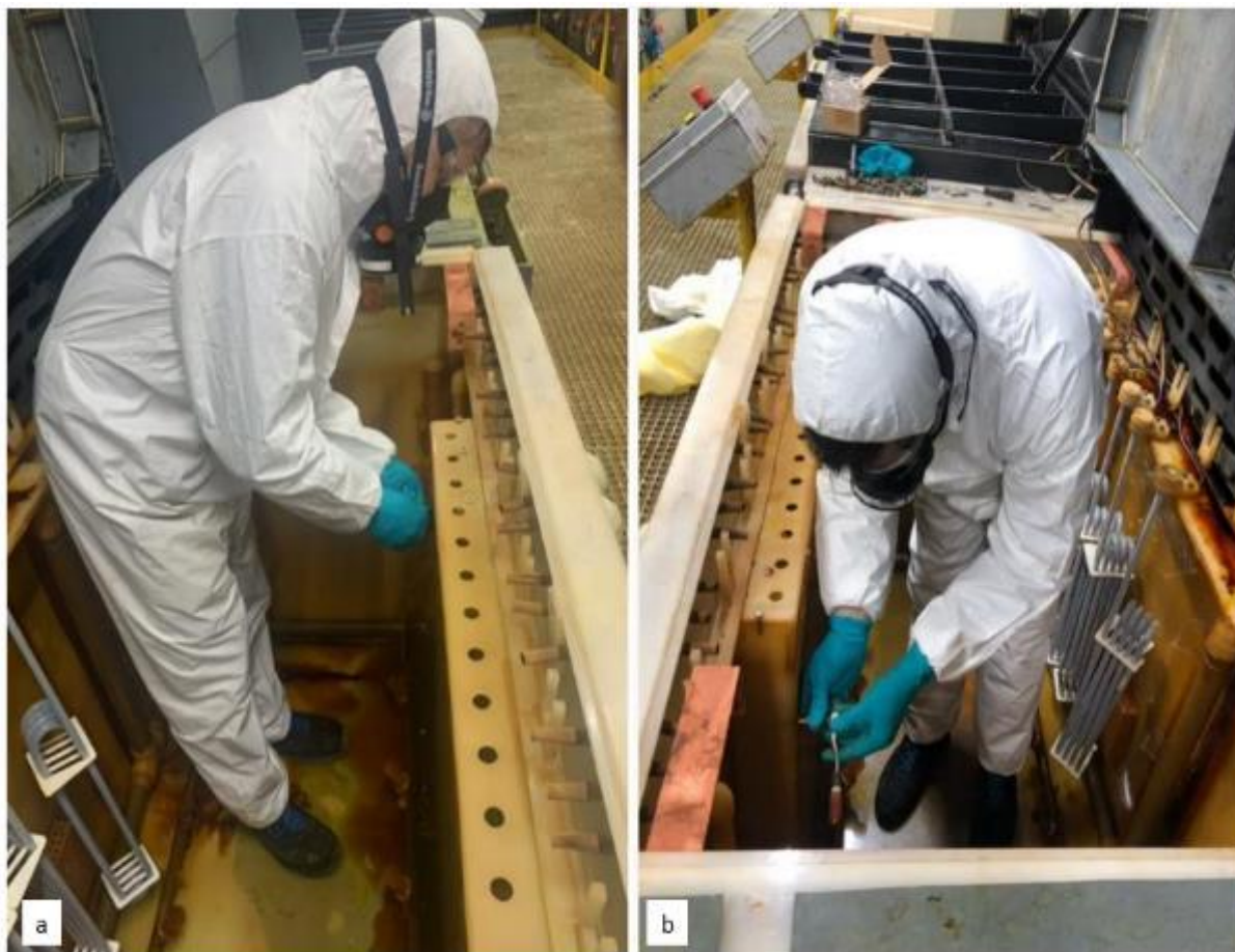
Figure 9-14: Cleaning of equipment (a + b)
