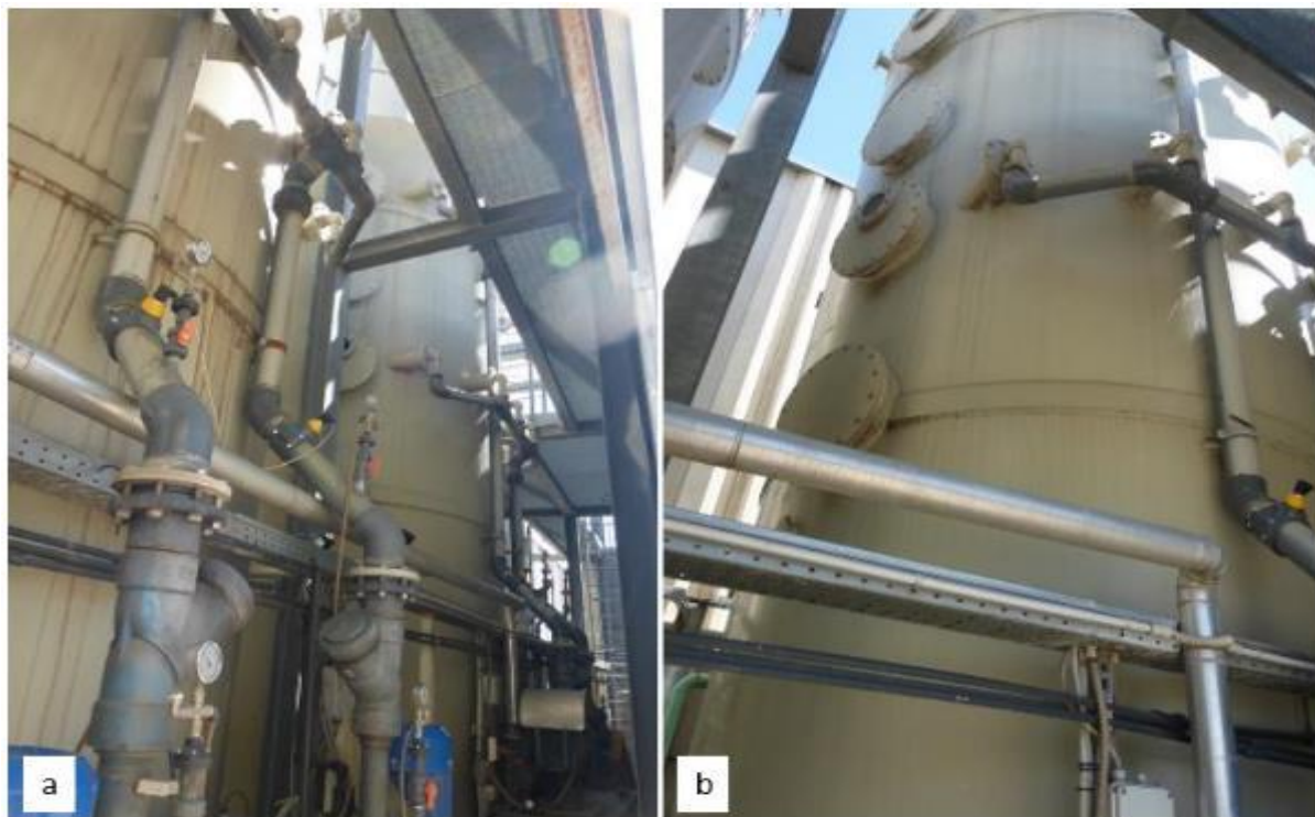
Figure 9-3: Wet scrubber (a + b)
