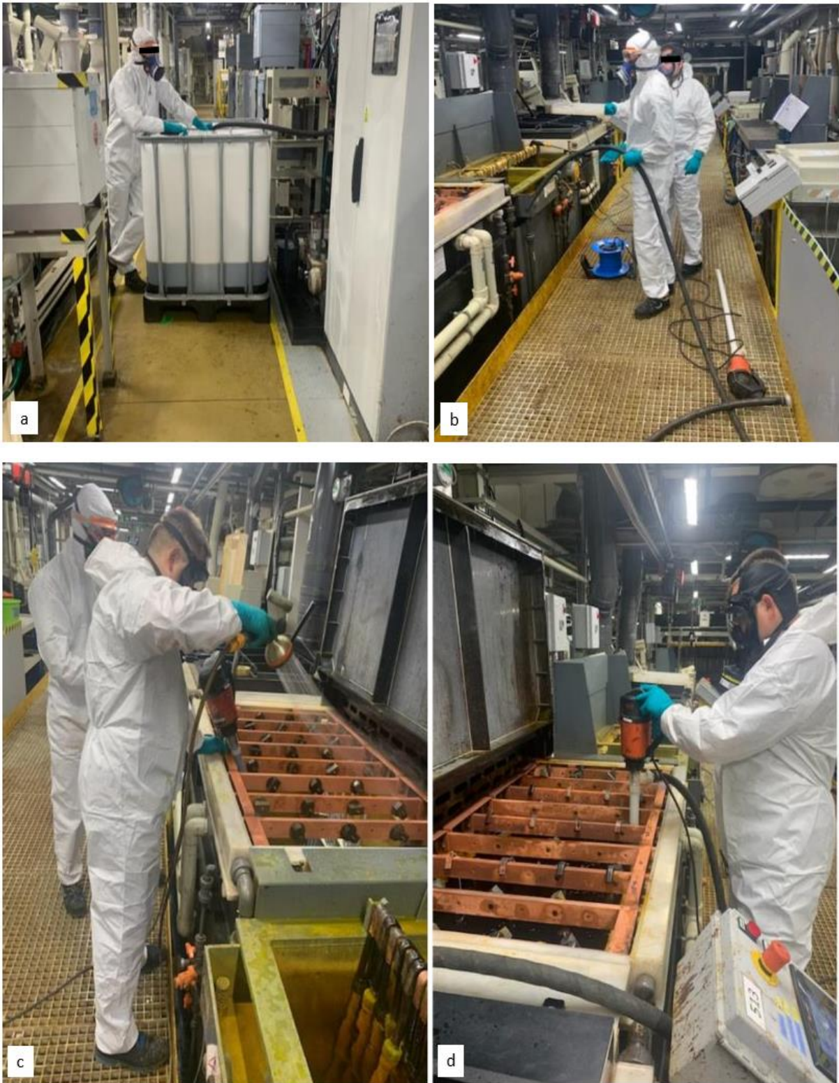
Figure 9-13: Bath emptying by transfer of old bath solution into an IBC (a) and bath cleaning with a hose and wet and dry vacuum cleaner (b, c, d)
