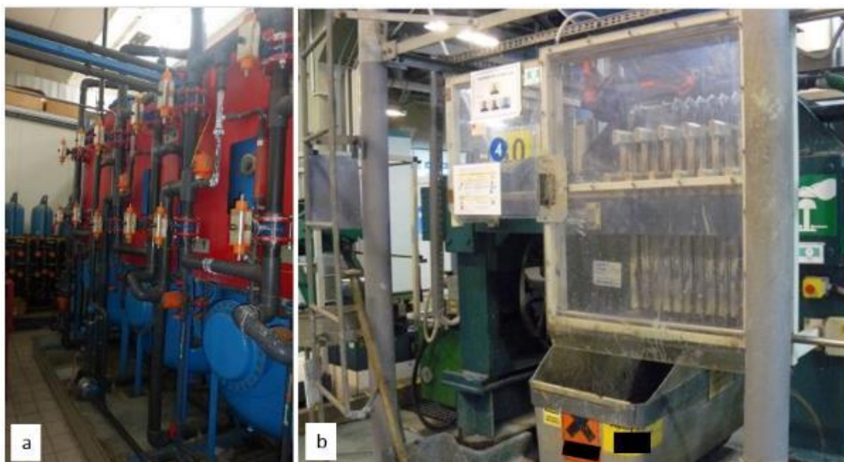
Figure 9-5: Water deionisation tanks for wastewater treatment (a) and filter press for separation of the filter cake (b)
