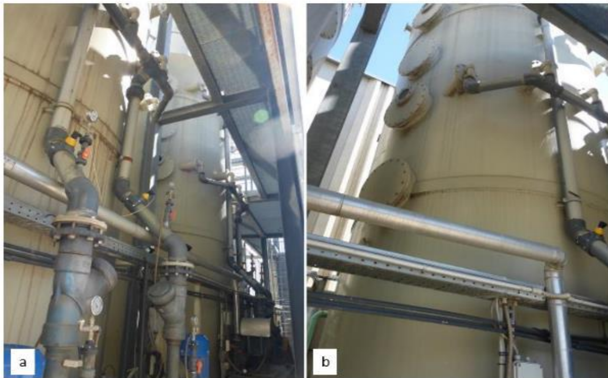
Figure 9-4: Wet scrubber (a + b)
