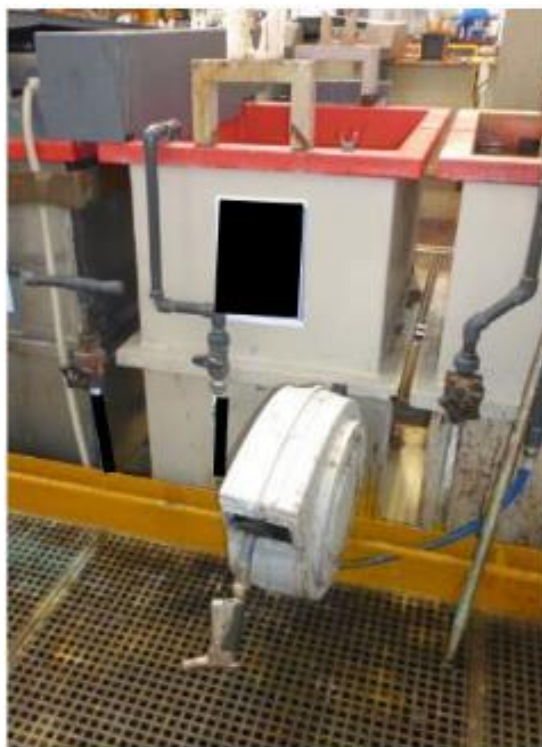
Figure 9-8: Hose for cleaning the edges of the tanks and the walkways surrounding the baths
