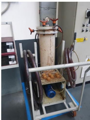
Figure 9-12: External filtering system
