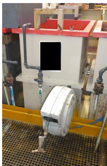
Figure 9-8: Hose for cleaning the edges of the tanks and the walkways surrounding the baths
