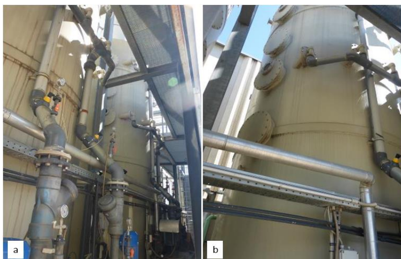
Figure 9-3: Wet scrubber (a + b)
