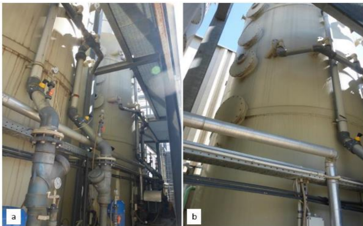
Figure 9-5: Wet scrubber (a + b)
