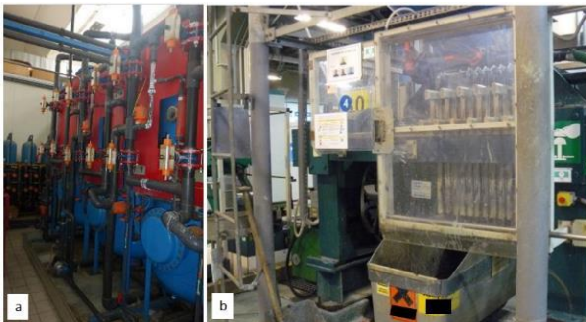
Figure 9-6: Water deionisation tanks for wastewater treatment (a) and filter press for separation of the filter cake (b)
