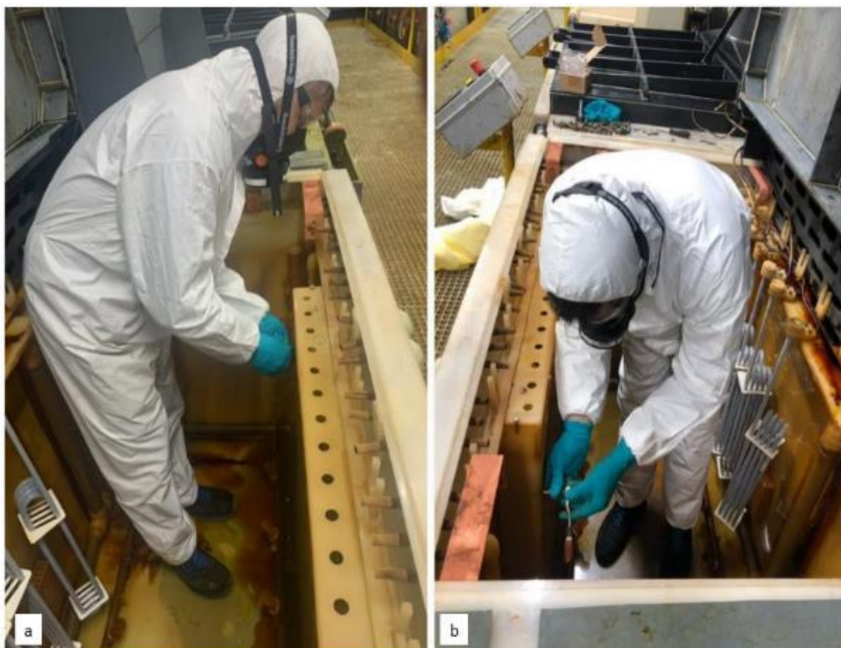
Figure 9-16: Cleaning of equipment (a + b)
