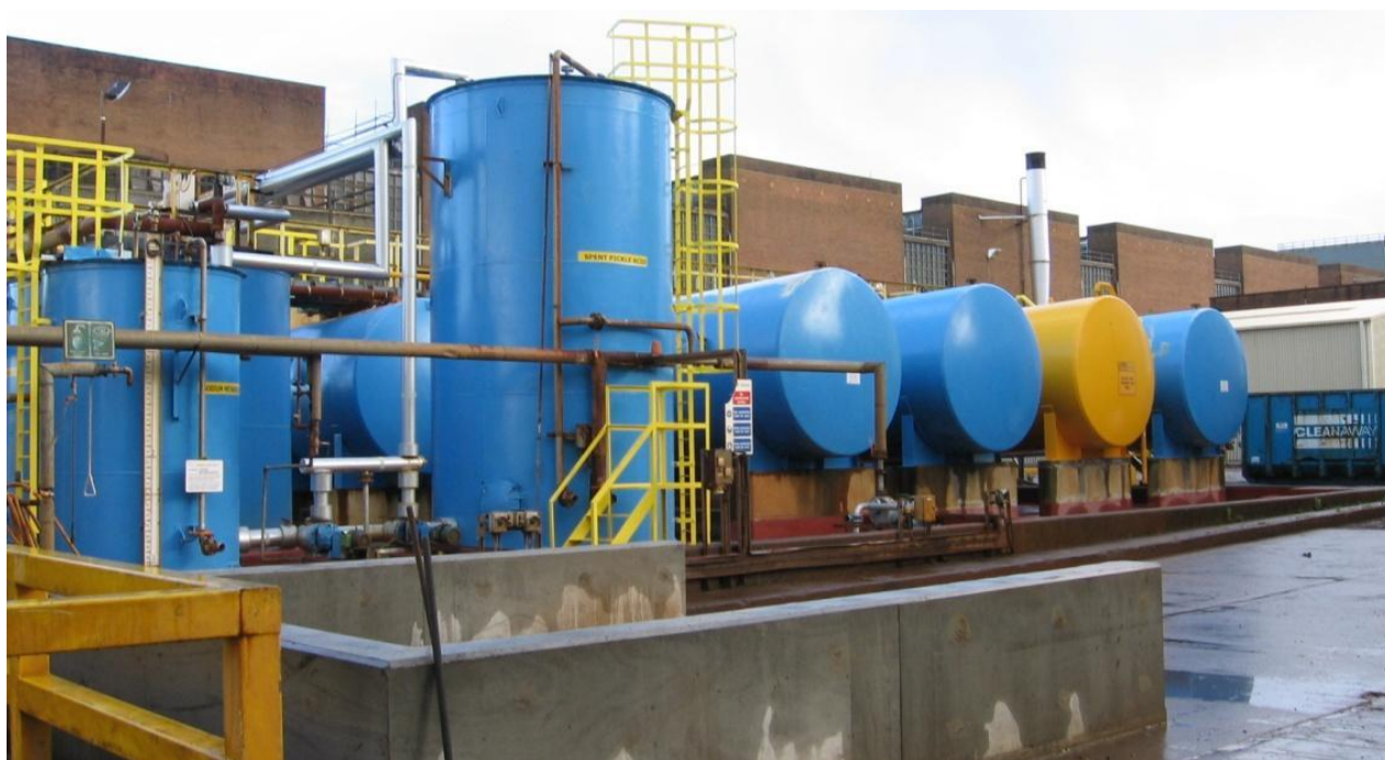
Figure 10: The tank farm in the WWTP
