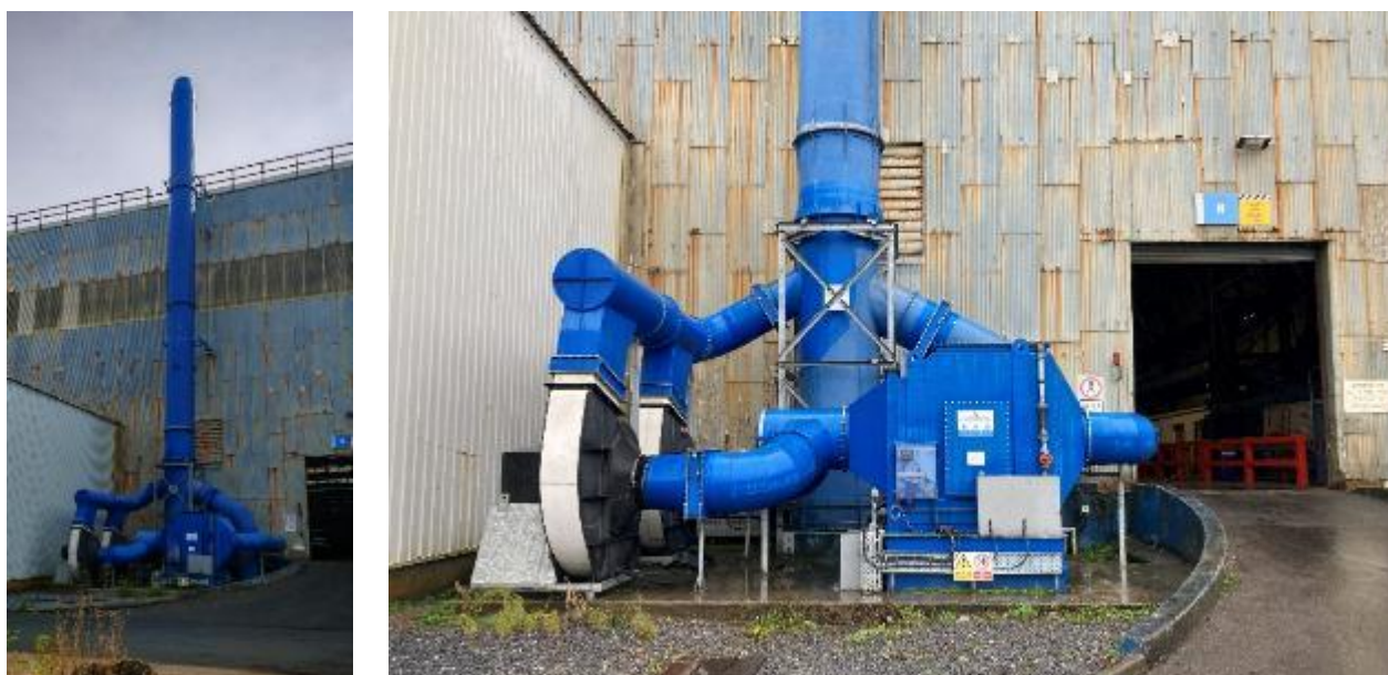
Figure 15: Stack serving the ETL5 line (L), wet scrubber attached to stack (R).
