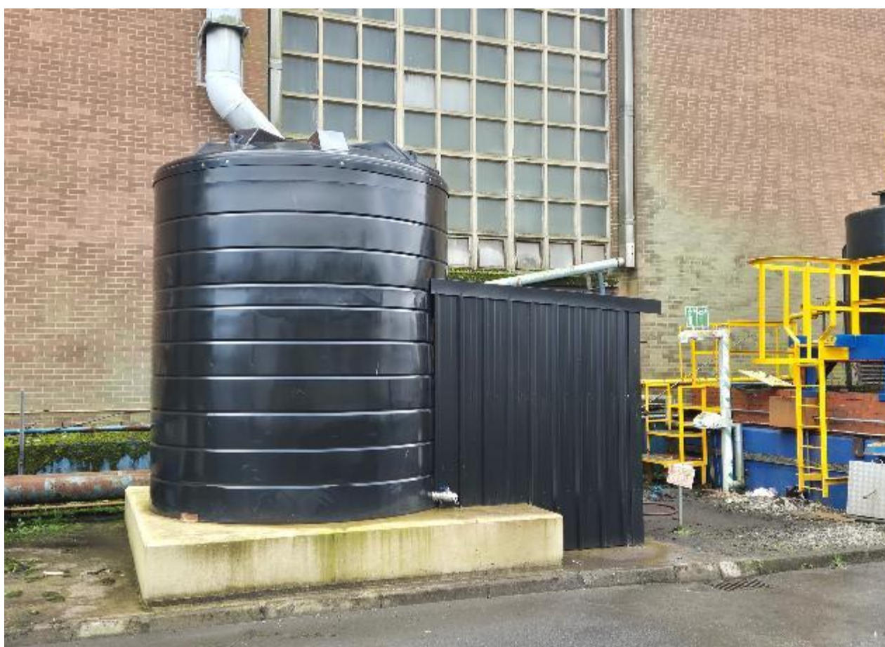
Figure 8: New bulk storage tank for future supply of sodium dichromate solution
