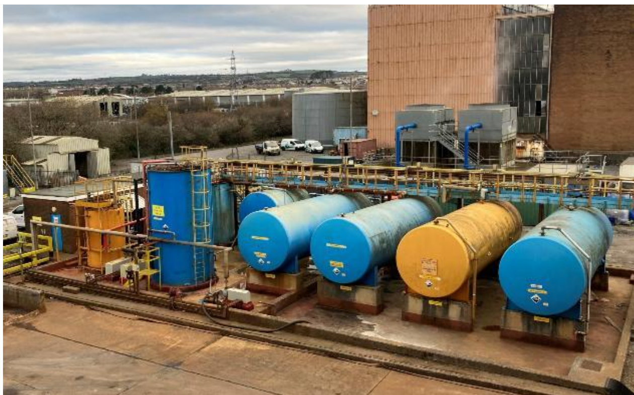
Figure 16: Tank farm in WWTP showing secondary containment (bundling)
