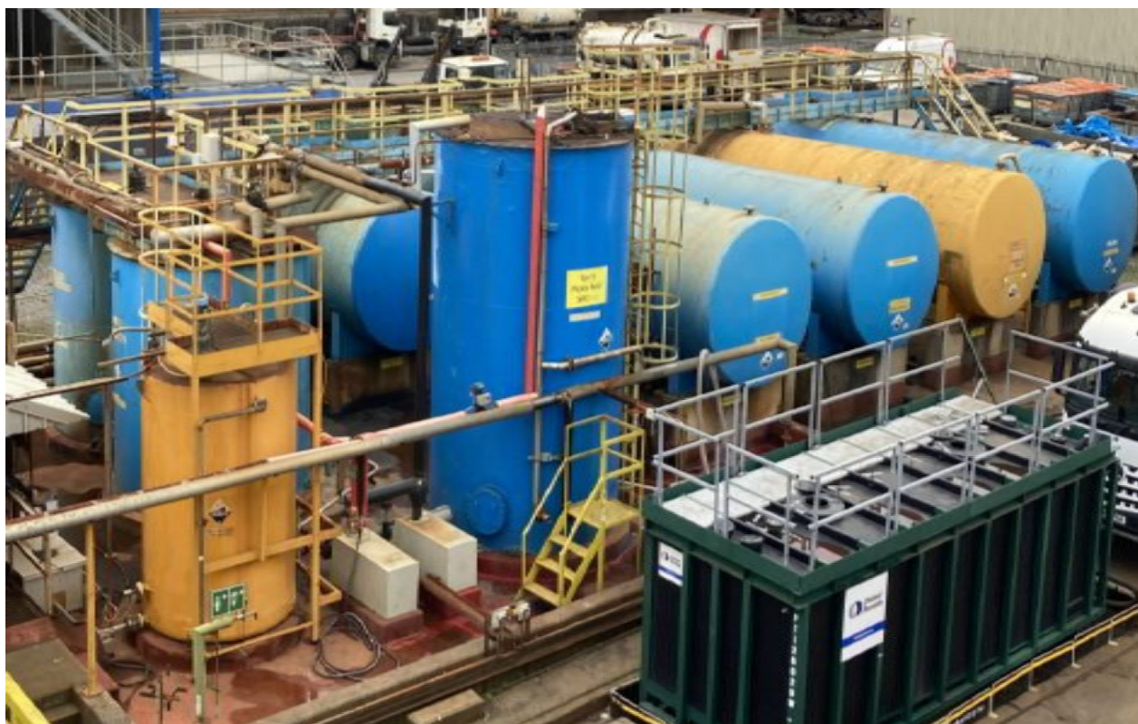
Figure 27: Bulk tank farm in the WWTP
