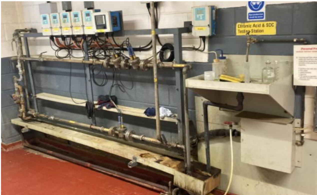
Figure 28: Testing station for chromic acid wastewater
