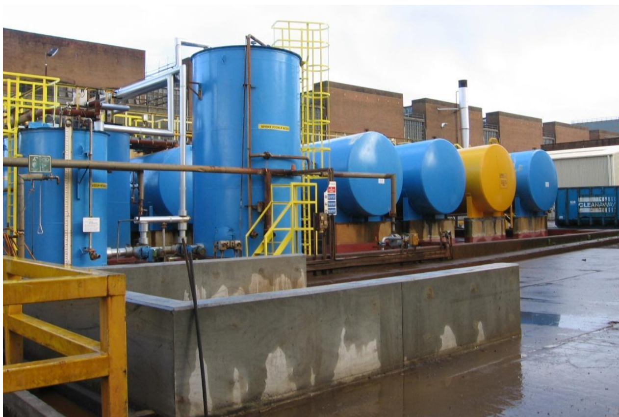
Figure 9: The tank farm in the WWTP
