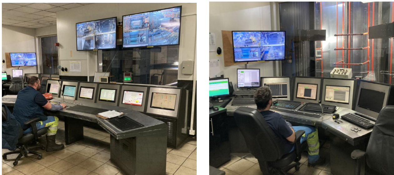
Figure 33: ECCS4 control room
