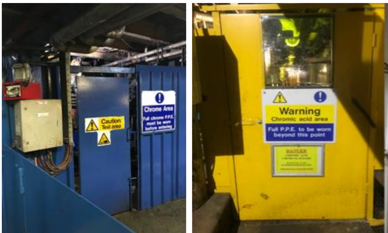
Figure 20: Segregated 'chromic acid area' in basement
