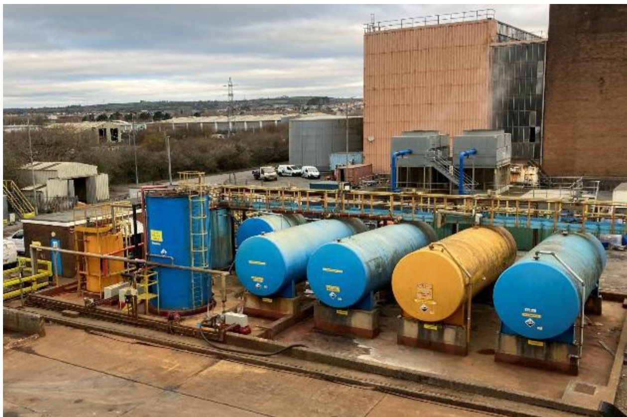
Figure 17: Tank farm in WWTP showing secondary containment (bunding)
