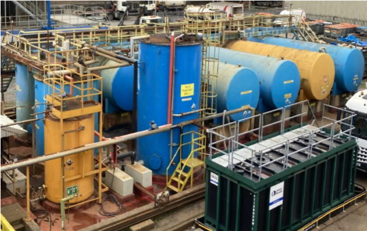
Figure 36: Bulk tank farm in the WWTP
