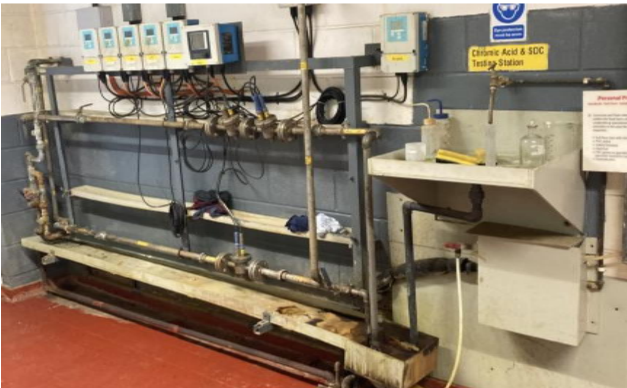
Figure 37: Testing station for chromic acid wastewater
